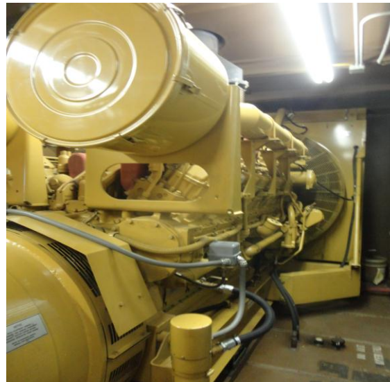
Caterpillar 1,275 kW Emergency Diesel Generator
