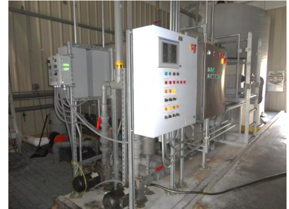
View of Waste Water Treatment System
