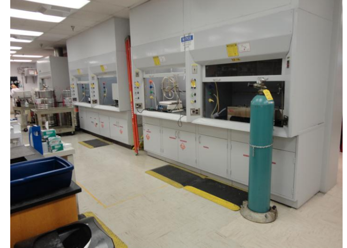
View of Fume Hoods
