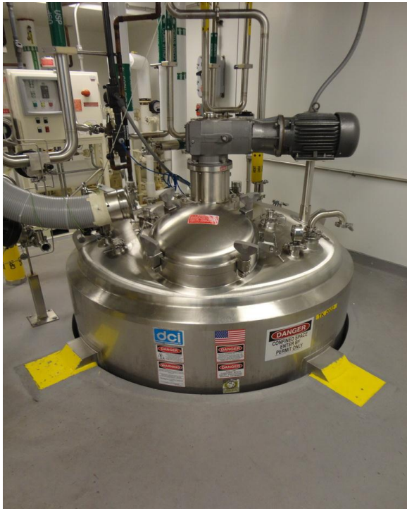
(1 of 4) DCI 1000 Gal Processing Tanks (2007)
