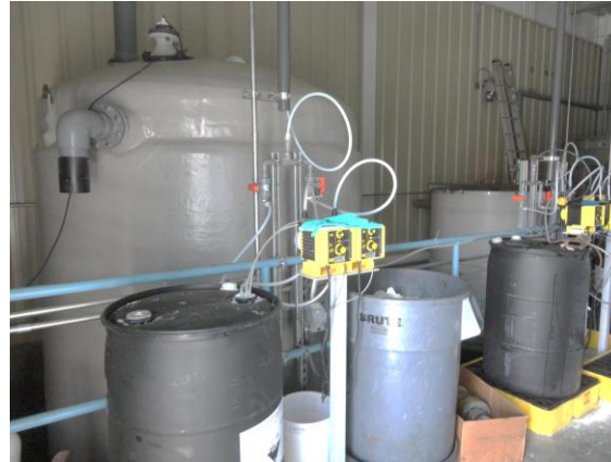
View of Waste Water Treatment System
