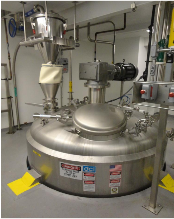
(1 of 4) DCI 2500 Gal Processing Tanks (2007)
