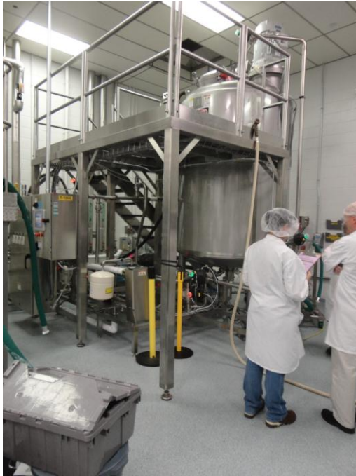
DCI 1,000 Gal Processing System (2012)
