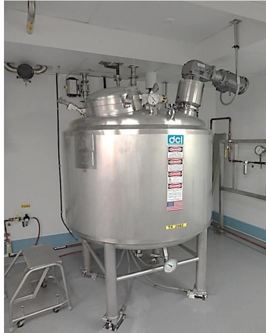
(1 of 2) DCI 250 Gal Processing Tanks
