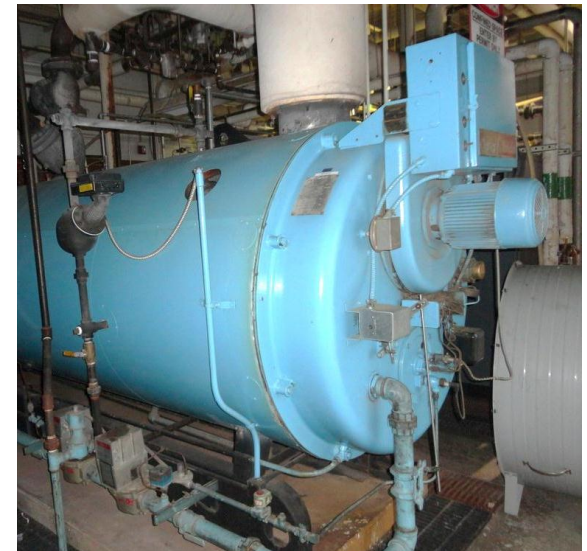
(1 OF 2) Packaged Steam Boilers
