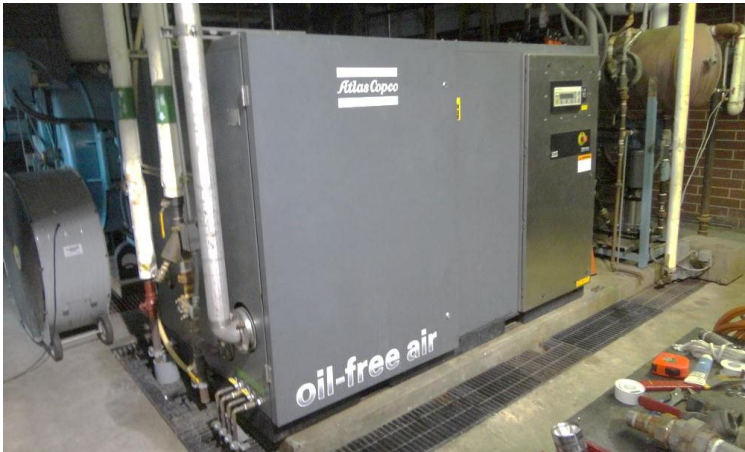
(1 of 2) Atlas Copco Oil Free Air Compressors (200HP & 150HP)
