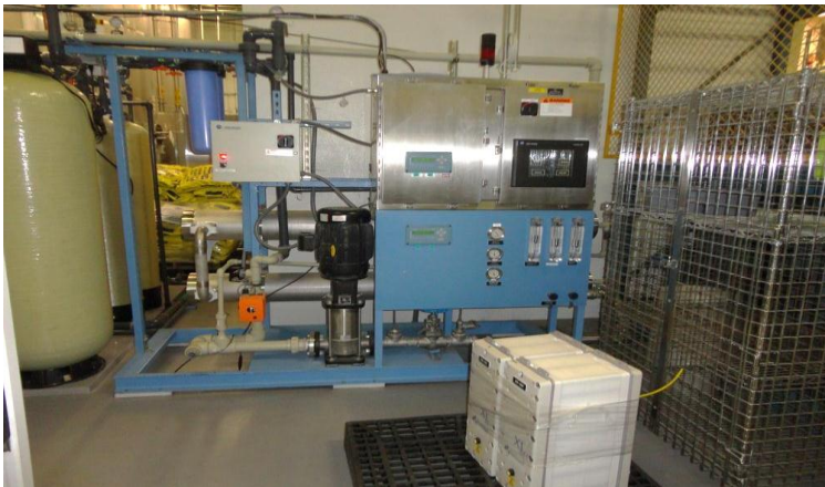
USP Water System with RO Skid, Ozone Skid and DCI 2,500 Gal Tank
