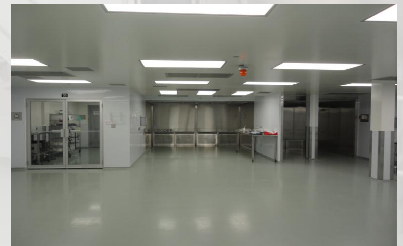
View of Raw Materials Process Area including HEPA Stainless Steel Extract Booths
