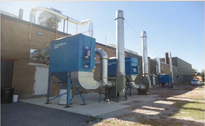
View of Torit Dust Collectors
