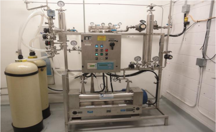
Purified Water System
