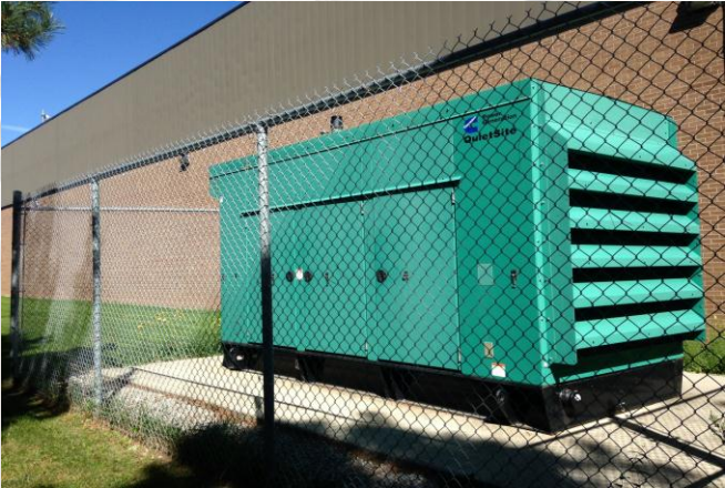
Cummins 400 KVA Diesel Fired Backup Generator
