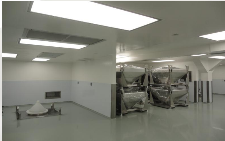
View of Second Floor Bin Handling and Dispensing Area Above Tablet Presses
