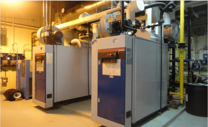
Dual Miura Gas Fired Boilers
