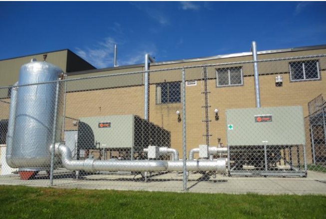
View of (2) Trane Chillers for Plant Air & Process
